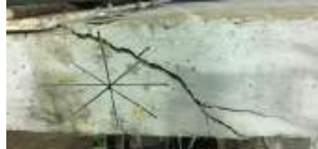
3.d) Final crack pattern of specimen (B4)
