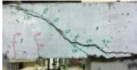
3.g) Final crack pattern of specimen (B7)
