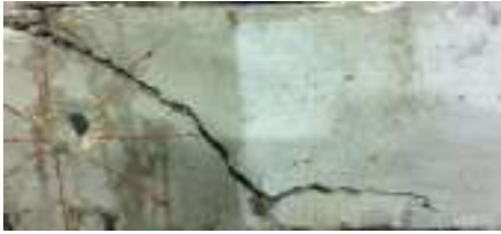
3.e) Final crack pattern of specimen (B5)
